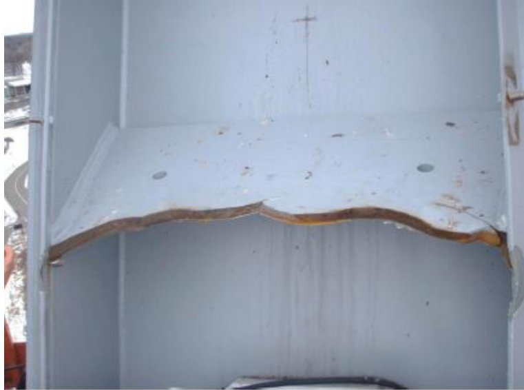
View of Cable Diaphragm Plate 9 after fracture.
