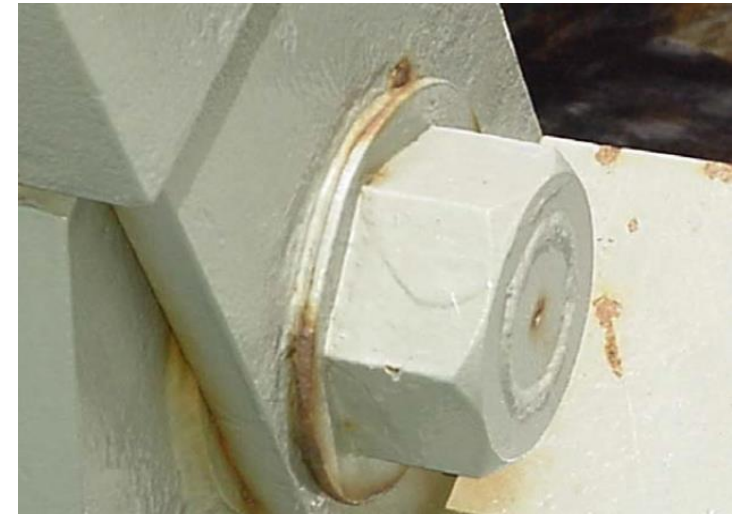
Possible over-tightened nut or crevice corrosion causing distortion of washer.
