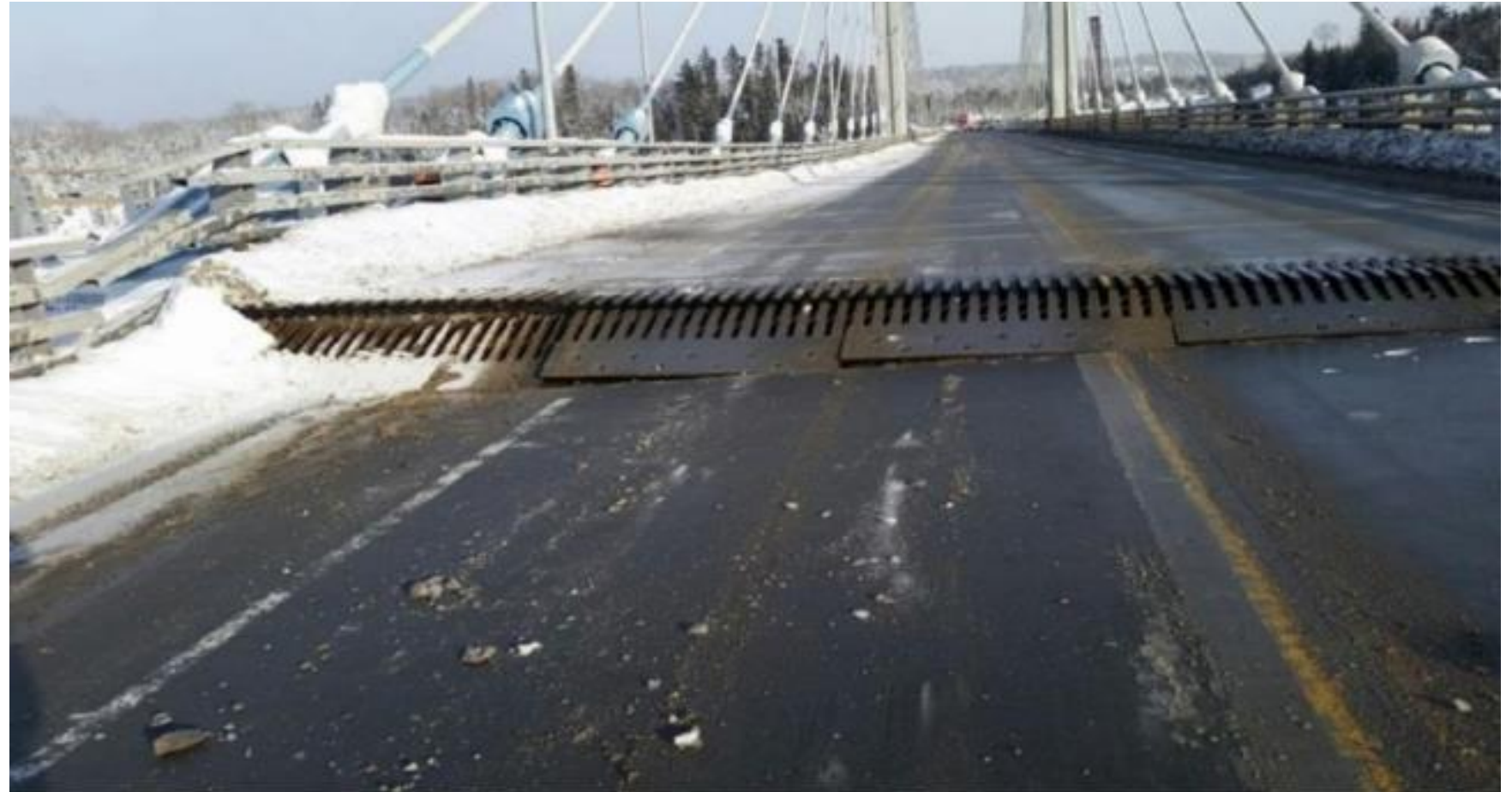
Nipigon River Bridge, 600mm uplift of north bridge edge at west abutment, January 10 th , 2016
