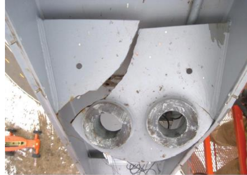
View of Cable Diaphragm Plate 8 following fracture and removal of Cables 8L and 8R.
