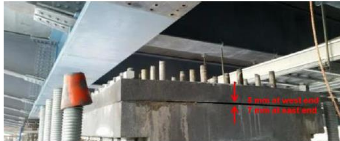
The observed permanent deformation of the shoe plate immediately after the failure of the bearing
