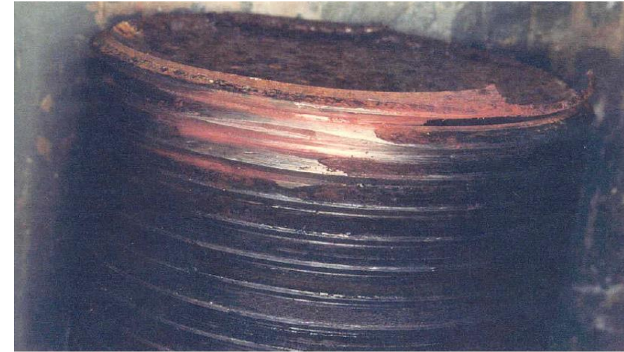
Hanger 1 (NW) – Shiny Area - Ground down threads.
