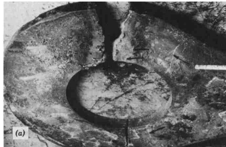
Cracked eyebar showing forge laps on the eyebar surface (courtesy of Santa Fe Railroad).
