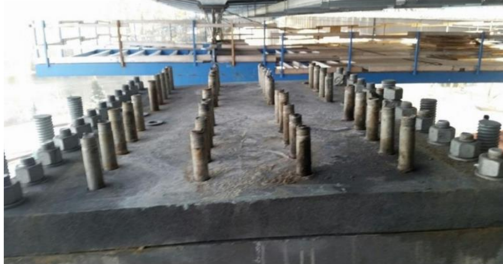
Fractured bolts (ASTM A490 bolt - connecting shoe plate to girder flange) and deformed shoe plate at north-west bearing. Note four lines of failed flange connection bolts.
