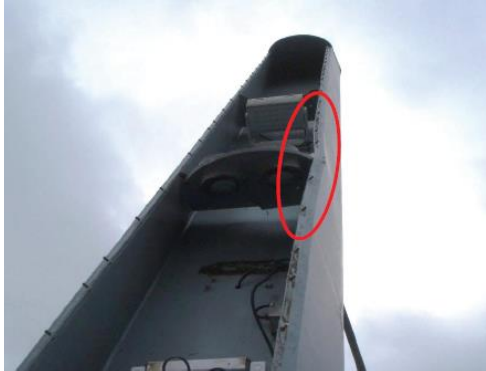
View of the left pylon flange alignment following local plastic rotation of the flange at the attachment elevation for Cable Diaphragm Plate 8.
